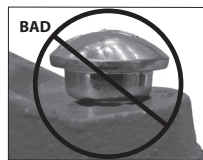
OVAL NECK OF BOLT NOT SEATED PROPERLY
