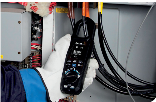
Verify amperage measurements
