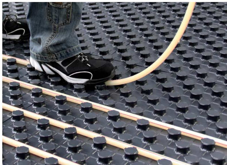
The Roth floor heating and cooling system at the State Museum Lower Austria, St. Pölten, Austria
