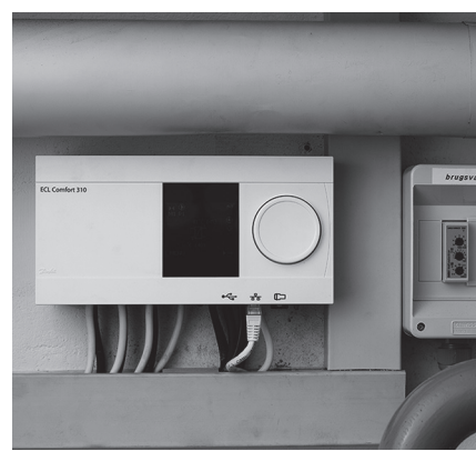
District Heating Controls
