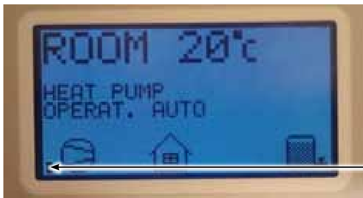
The image shows an open operating pressure switch or too high discharge pipe temperature
