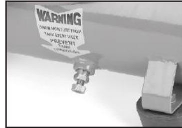
Tank drain valve.
