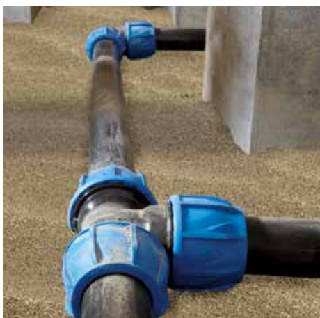
Water Distribution Lines
