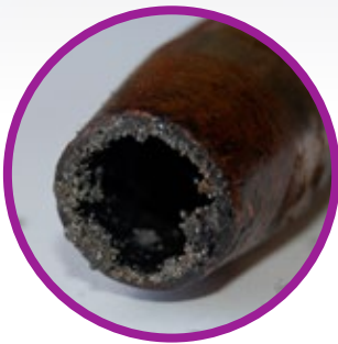
WITHOUT PROTECTION, AFTER WELDING
